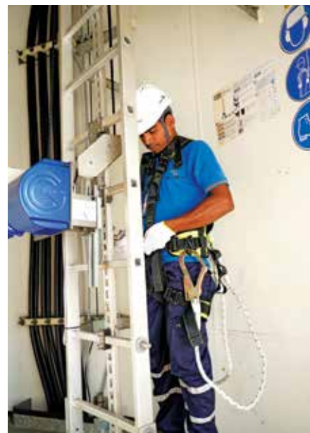
Safety harness for fall protection at our wind power plants
