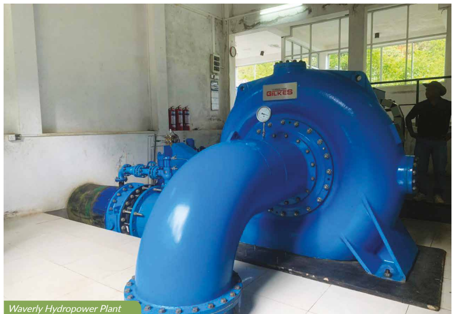
Waverly Hydropower Plant
