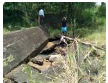
Pre-condition of the tank's spill
