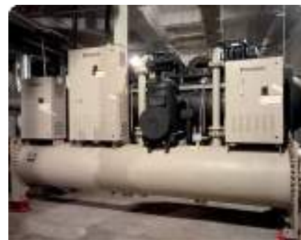
'Smart Technology Magnetic Bearing Chiller' placed at the Bank's Head Office
