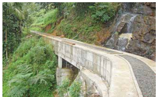
Drainage system to allow natural water paths to flow to the river
