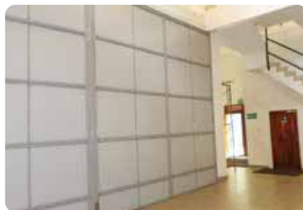
Noise control panel Installed at Erathna MHP
