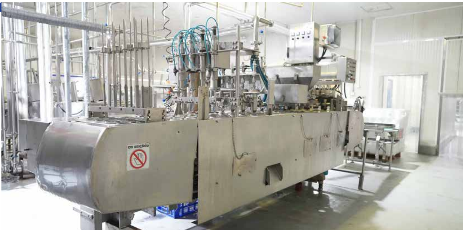
UHT Storage in Banduragoda Dairy Factory
