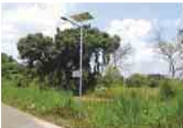
Solar powered street lighting
