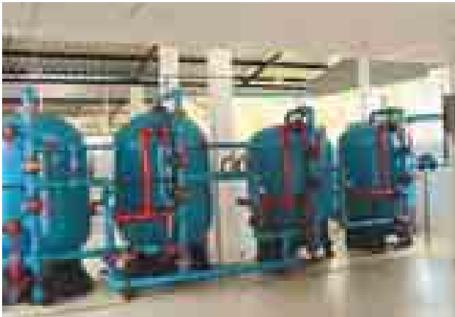
Water treatment plant at Cinnamon Lodge Habarana
