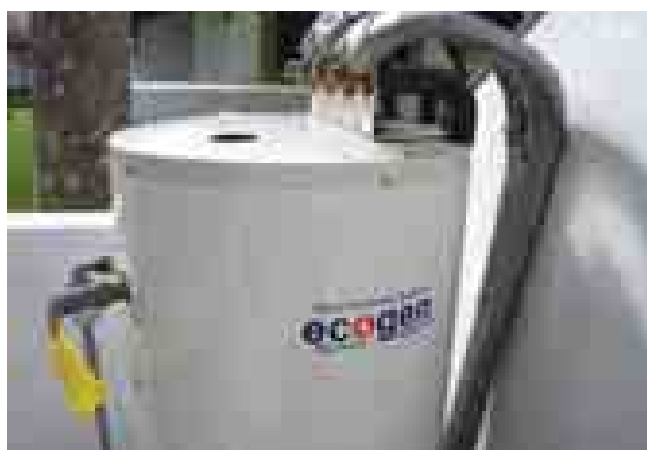
Ecogen water heating at Cinnamon Lodge Habarana
