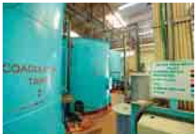
Water treatment plant at Ceylon Cold Stores
