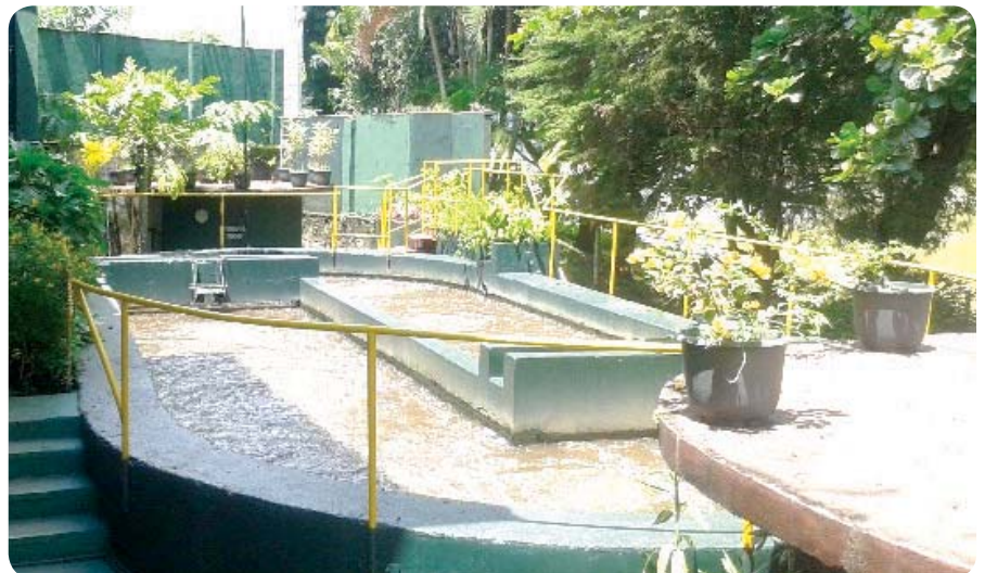
Effluent Treatment Plant at 'Cinnamon Citadel Kandy'.
