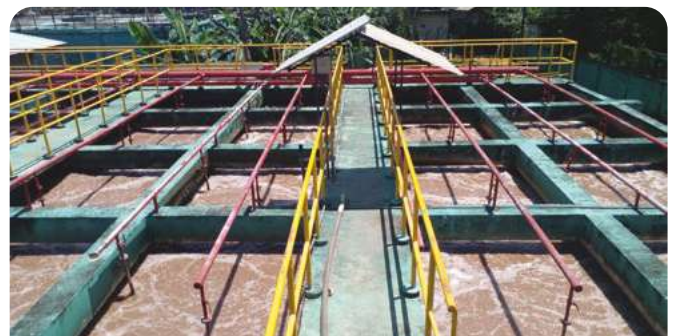
Effluent Treatment Plant at Ceylon Cold Stores.
