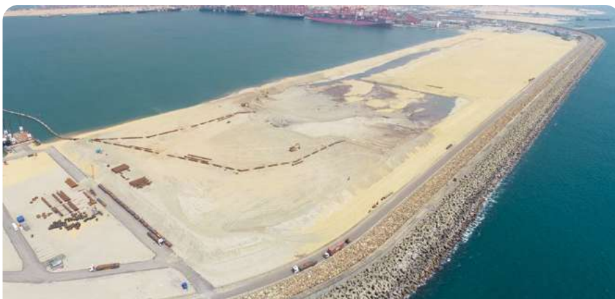
The entirety of the dredging works for both phases at WCT-1 is near complete.
