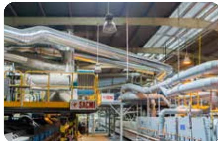
Reusing of waste heat through modern heat recovery system
