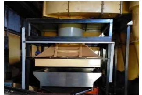
New Steam boiler in Dunsinane Estate | investment of LKR 19.6Mn..
