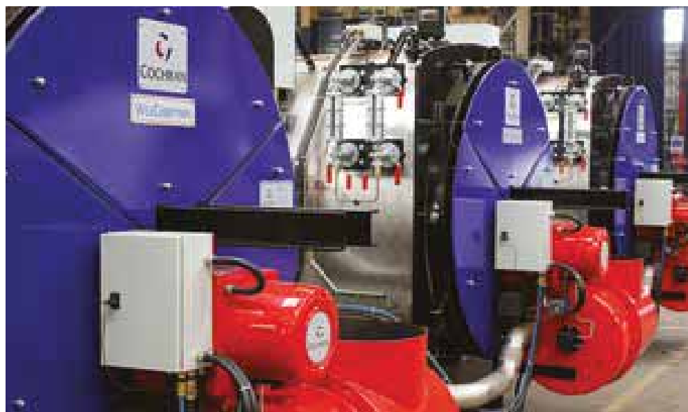
A Cochran Boiler Machine fully operational at a plant
