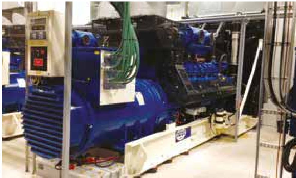
Fully operational FG Wilson Generator at site
