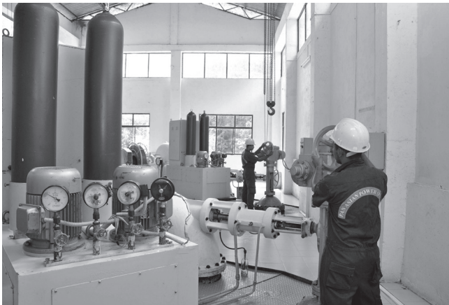
2 Mw Rathganga Hydro Power Plant
