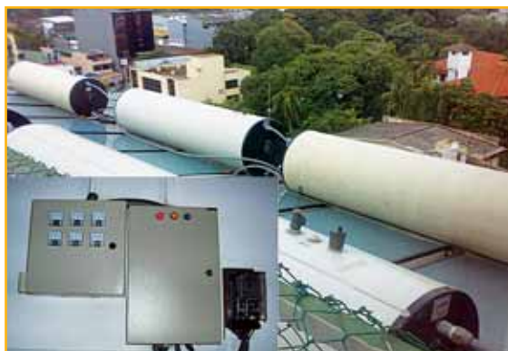
Hot Water Solar Unit
